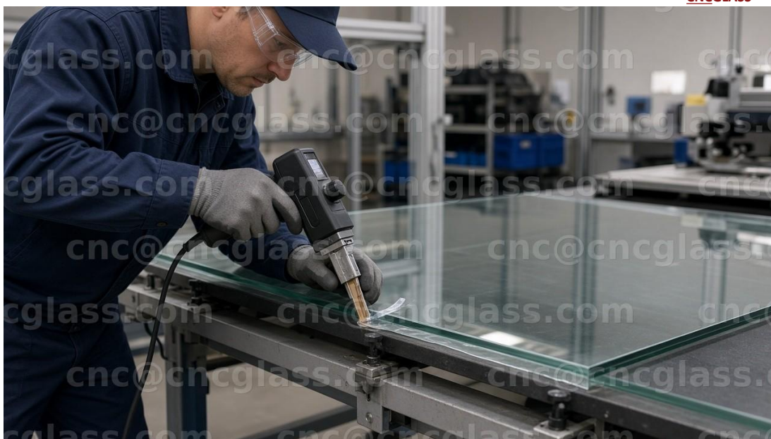
Figure 4 — Remediation: thermal cutter removes overflow that still appears after lamination.
